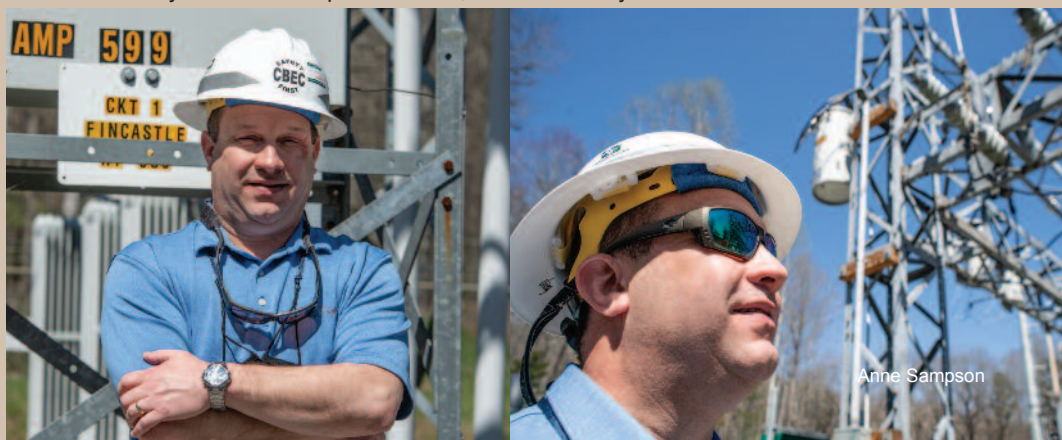
Jeff surveys the Coal Gap Substation, constructed by the CBEC in the mid-70’s.
